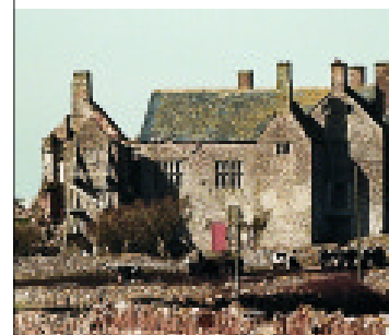
Tŷ'r Sgêr, ger Porthcawl. Uchod: Cyn y gwaith atgyweirio (Hawlfraint: Buildings at Risk [John Chapman Photographic]). Chwith: Gwneud y gwaith.
