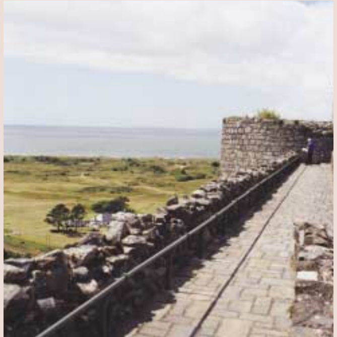
Safety railings (above) at Harlech Castle, designed to comply with safety regulations without being visible on the skyline of the castle (opposite).
