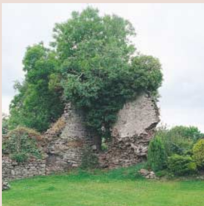
The precinct wall, before (below) and after (above) conservation work. Opposite: The restored well.
