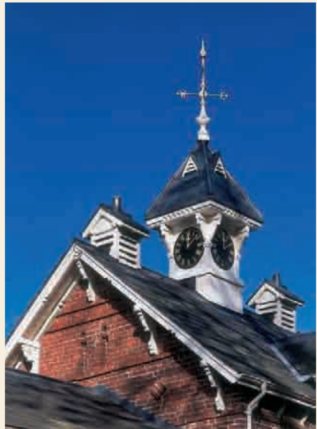
A view of the roof of an outhouse at Drybridge House before (left) and after (above) restoration.
